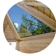
Roof window is not opening. The glass is clean and tempered, 8 mm thick.
